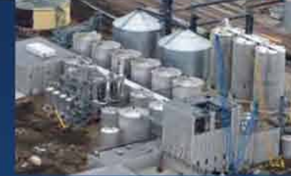
23 Field-Erected Tanks Casselton, North Dakota 18 Stainless Steel 5 Carbon Steel
