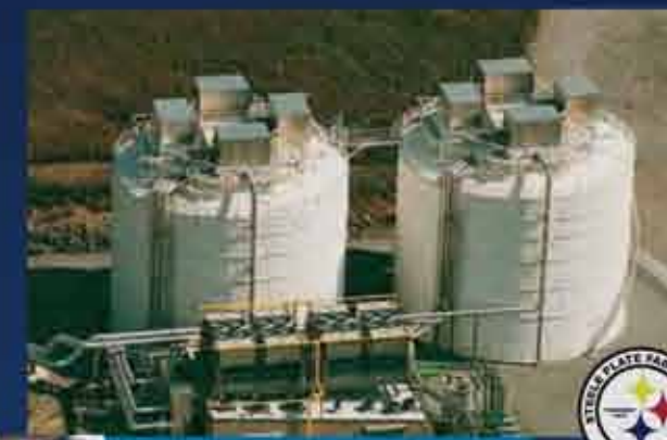
(2) 2,200,000 Gallon Ice Tanks Burgin, Kentucky Steel Tank of the Year 2000 - Steel Plate Fabricators Association
